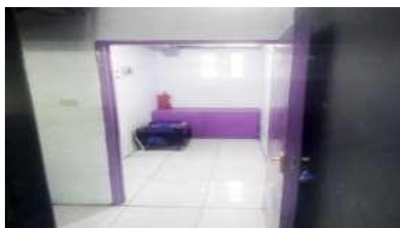
Fig 5. Inside View of the generator storage room
