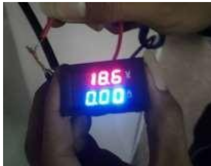
Figure 6. Solar Panel Measurement
